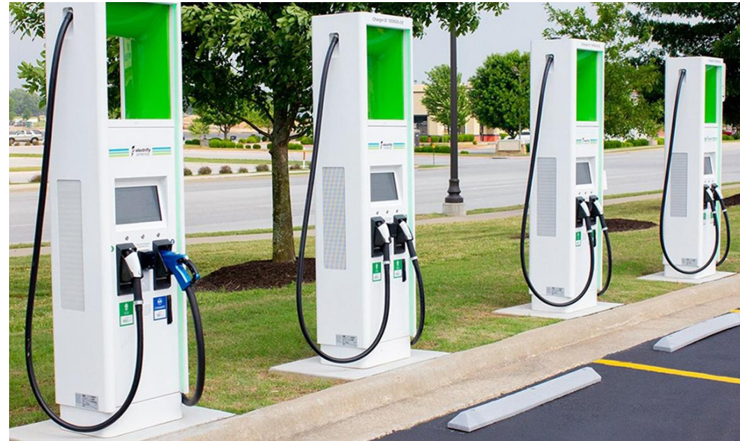
Figure 1: EV Charging Stations 1
