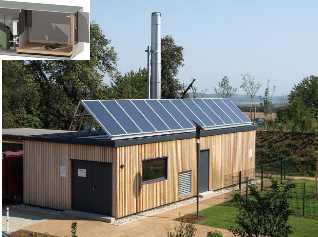
Containerised biomass heating cabins
