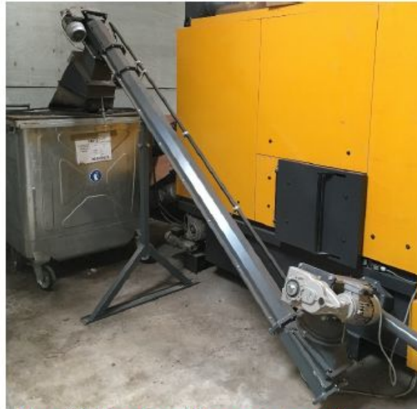
Figure 6.1: Conveying ash to a separate container within the boiler house
