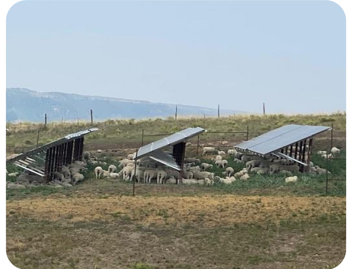
Last Dollar Solar Array
