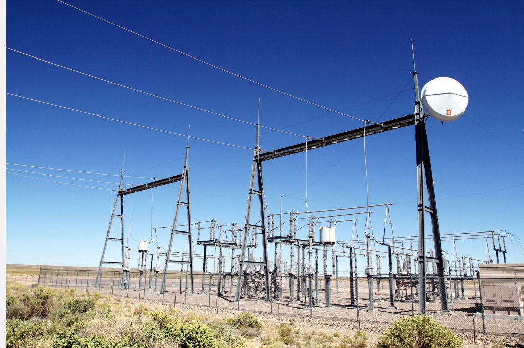
0-5 Miles from Substation
