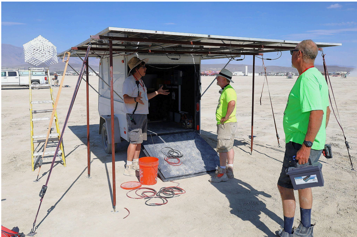
RAT's Darren Emmons, Bob Wolff, and Steven Queen at the RAT Solar Generator Trailer
