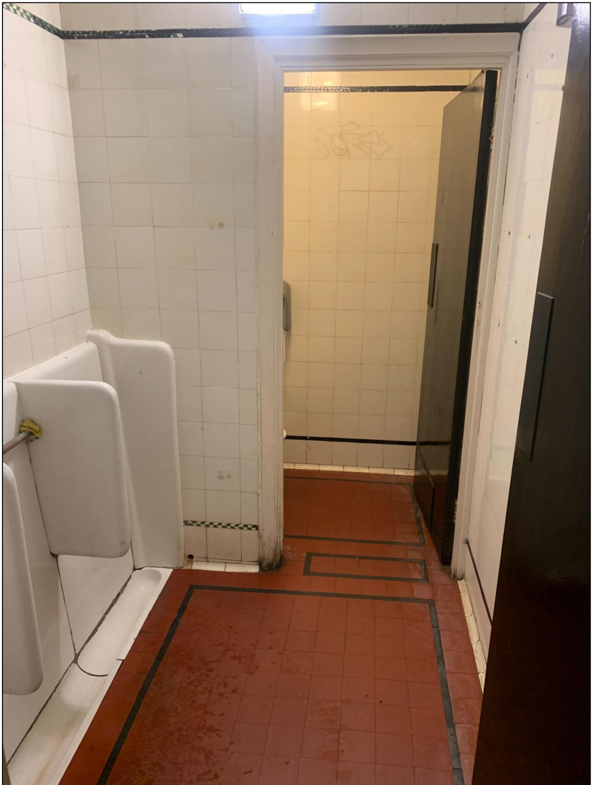
Toilet with urinals and stall
