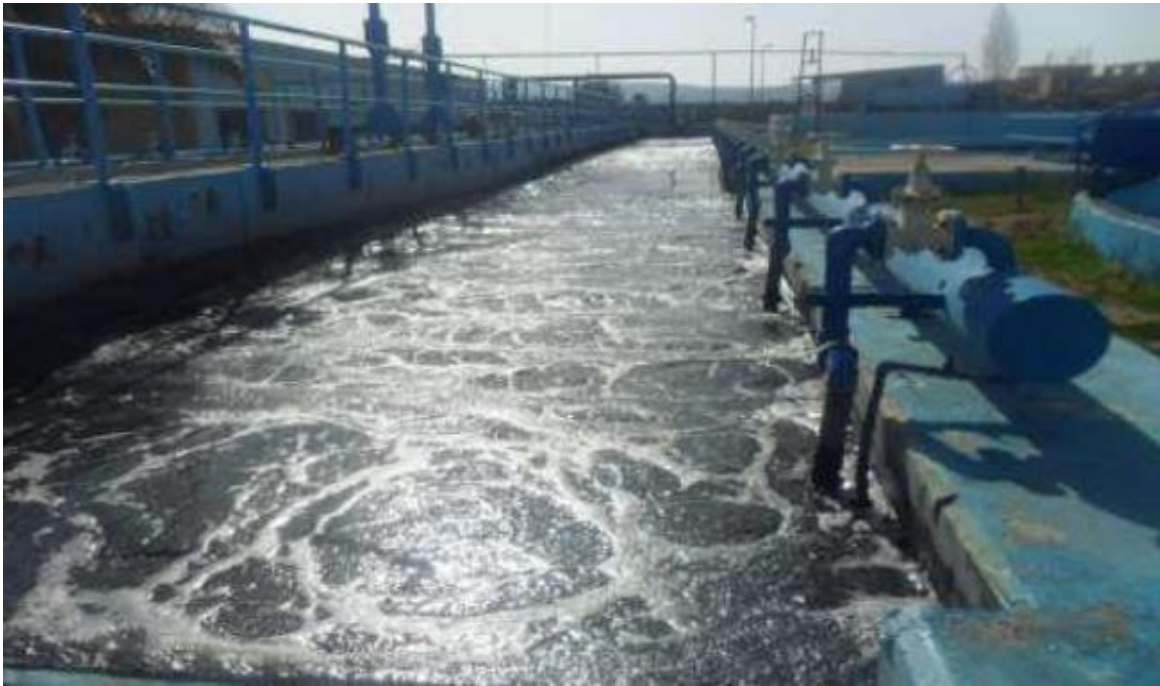
Figure 5. Biological basin (aeration basin).
