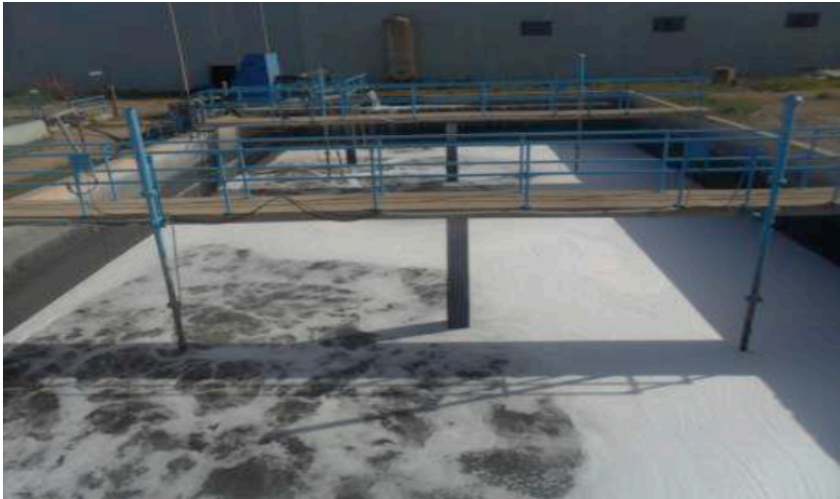
Figure 2. Photo of mixing and equalization basin N ° 1.
