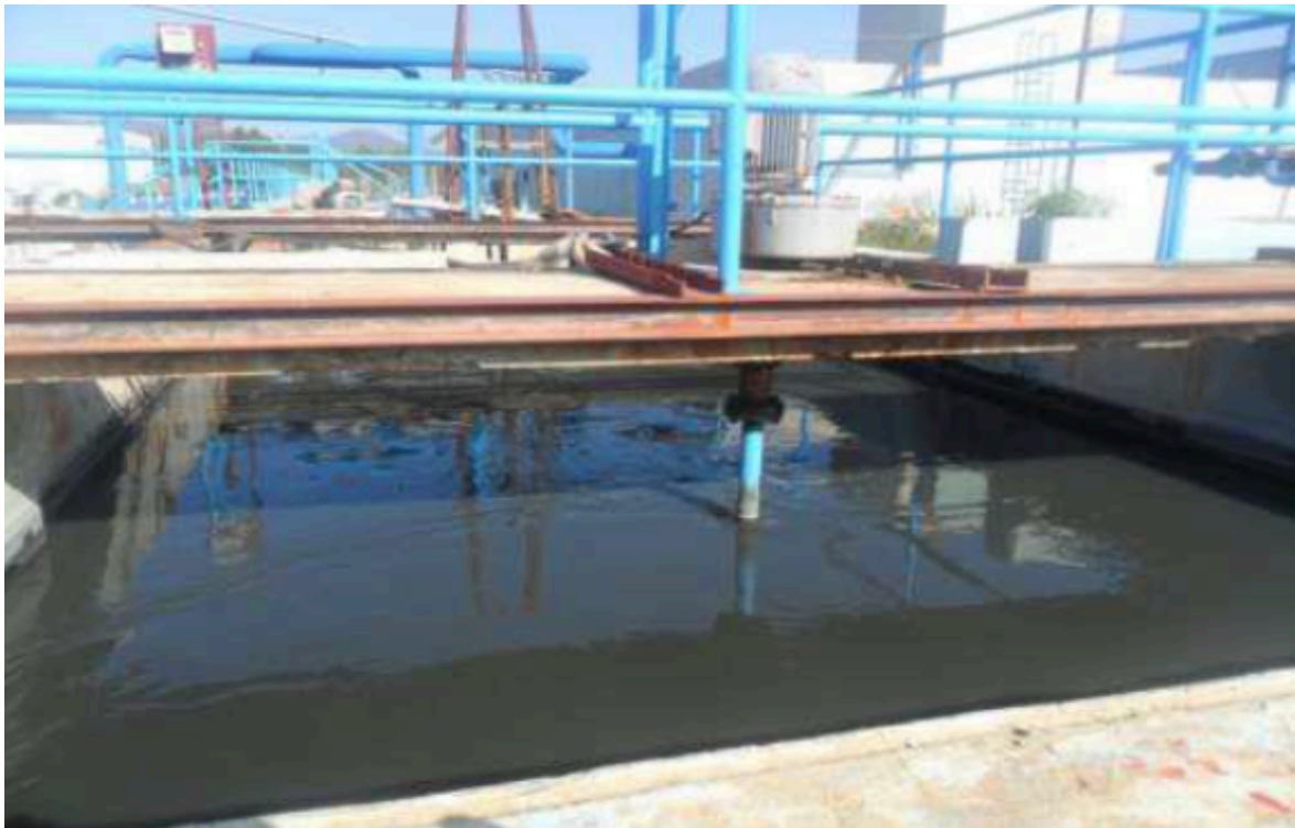
Figure 3. Mixing and neutralization basin N ° 2.
