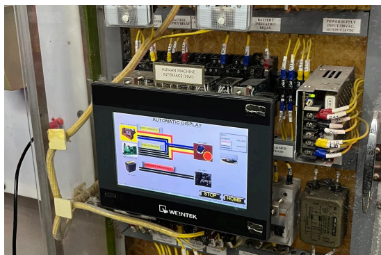
Gambar 4.5 Kondisi Running A Main Generator
