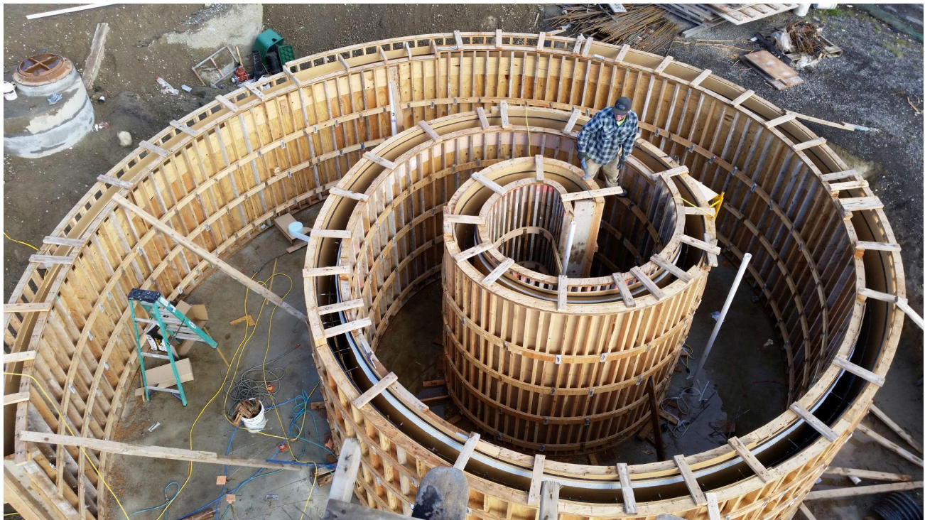
Construction of the spiral rain garden that is designed to treat low flows from groundwater and small storms to assist the larger treatment cells.
