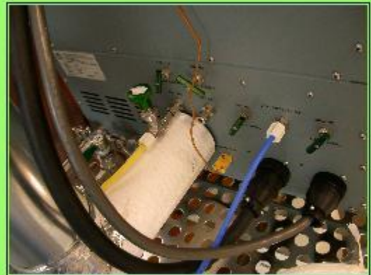
Hot and Cold N2 Flow Control Valves
