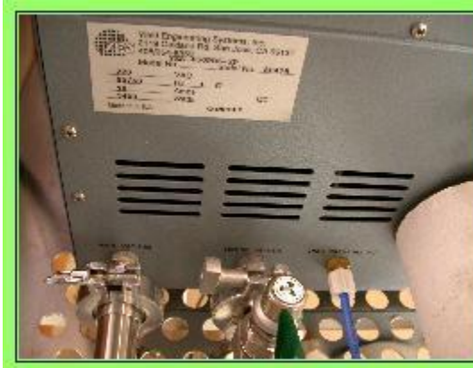
Main Vacuum & House Vacuum
