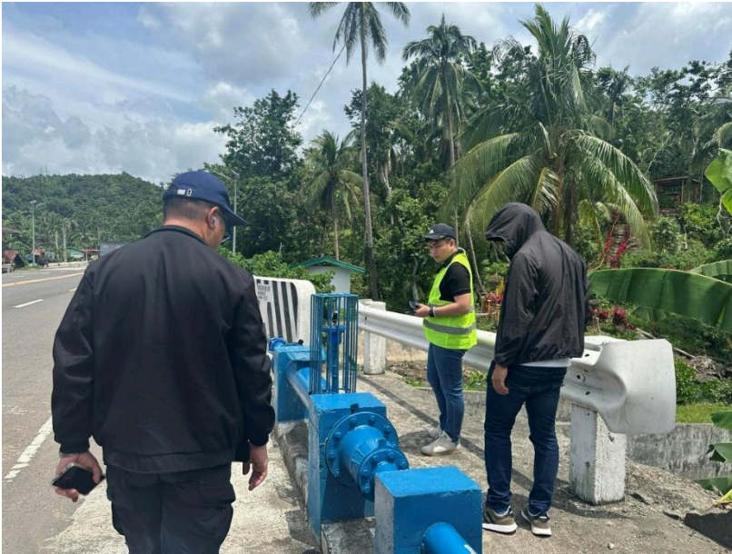
Figure 13 Inspection of the Booster Pump
