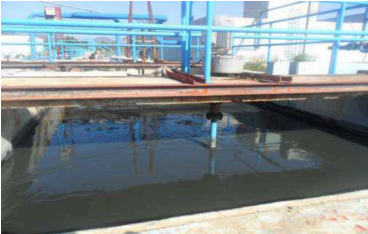
Figure 3. Mixing and neutralization basin N ° 2.
