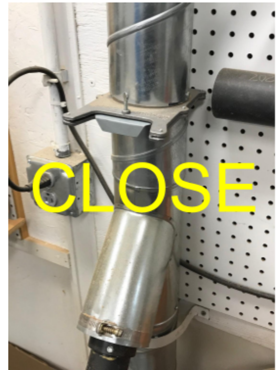
Fig. 11: Blast gate by vacuum hose
