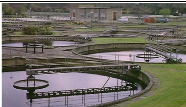
Example of Sewage Disposal (Nottingham Trent University, UK)
