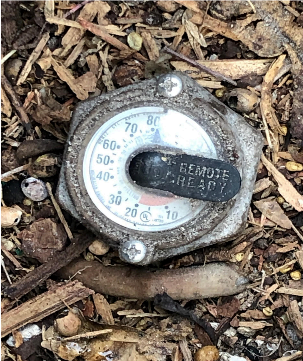
OKEECHOBEE GUARDHOUSE- EMERGENCY GENERATOR PROPANE FUEL SUPPLY CONFIRMED, APPROXIMATELY 400 GALLONS.
