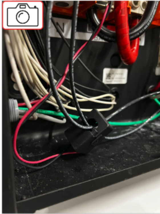
Meter Y Solar CT Monitoring Two PV L1 Circuits - CT Facing The Source Inverter
