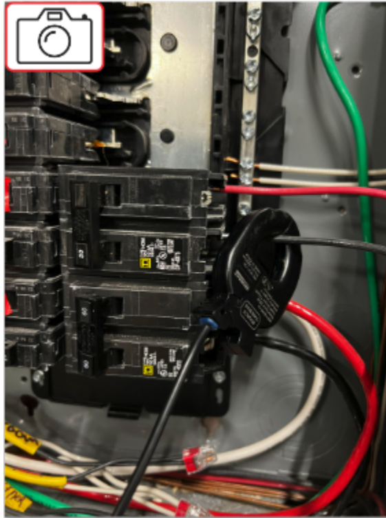
Remote Neurio Meter Monitoring PV L1 Circuit In MSP - CT Facing The Source Inverter
