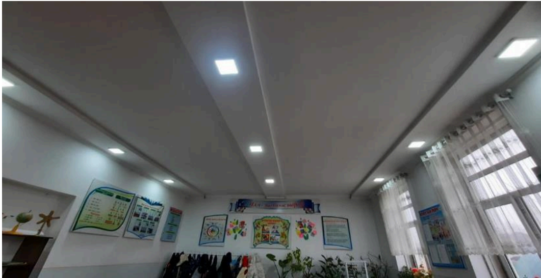
Photo 5. No ventilation system in classrooms
