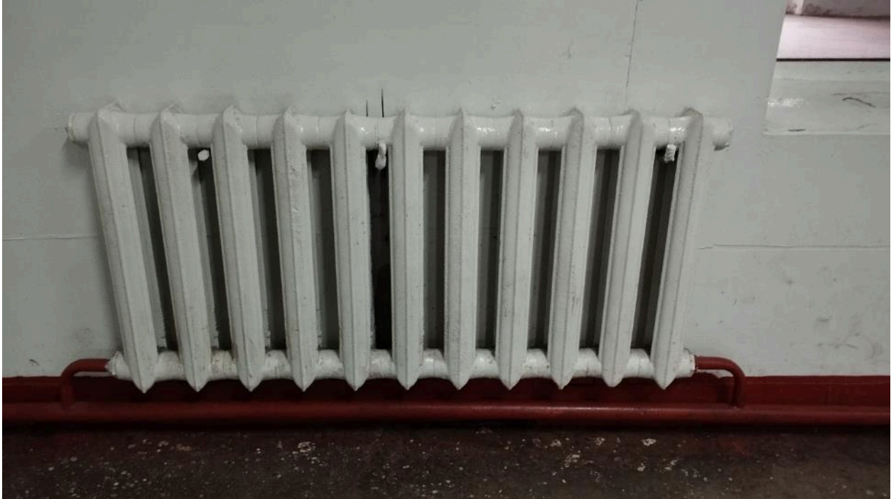
Photo 4. School heating system. MS-90 cast iron radiators.
