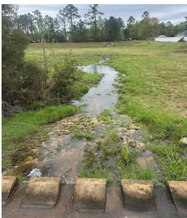
Figure 1: Current inlet conditions after a rainfall event
