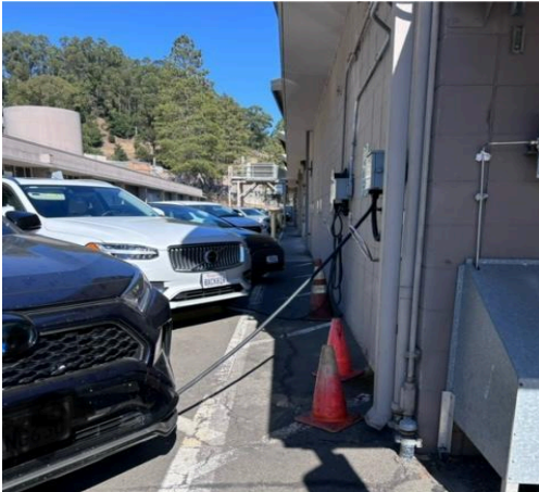
Incorrect cord draping across walkway
