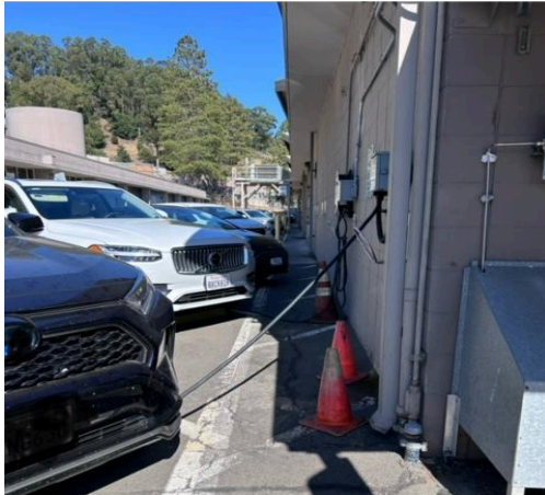
Incorrect cord draping across walkway
