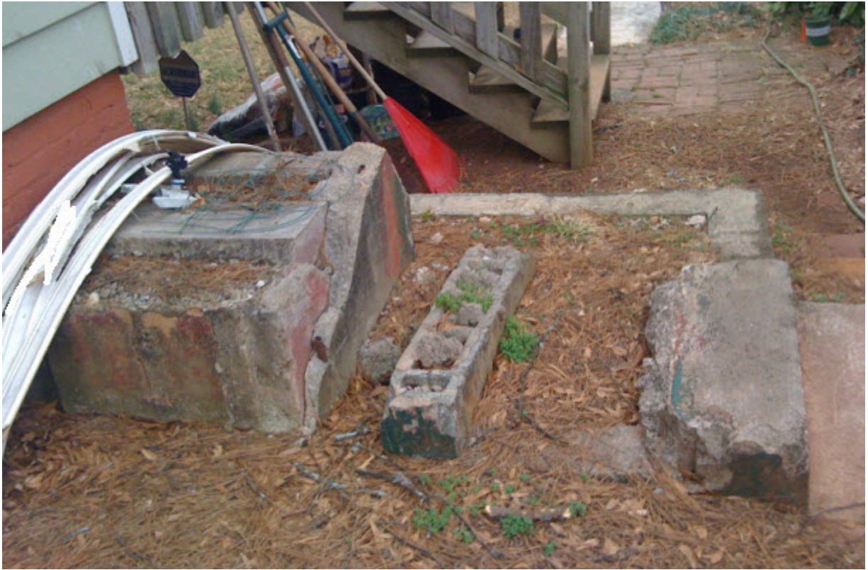
Figure 7: The stairway is old and full of rubble like this, but has less plant life
