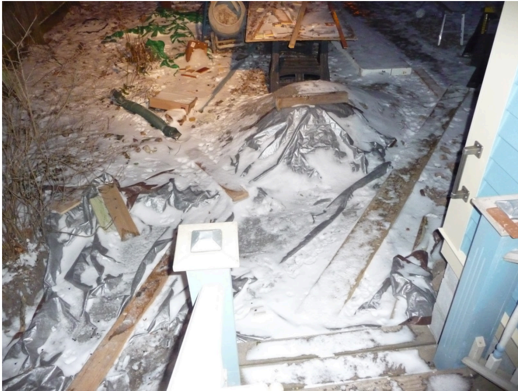
Figure 38: The area surrounding the stairwell is full of rubble
