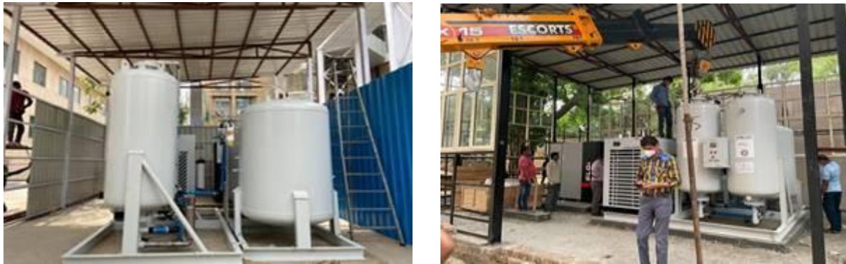
Fig 5: Medical oxygen plant at AIIMS New Delhi
