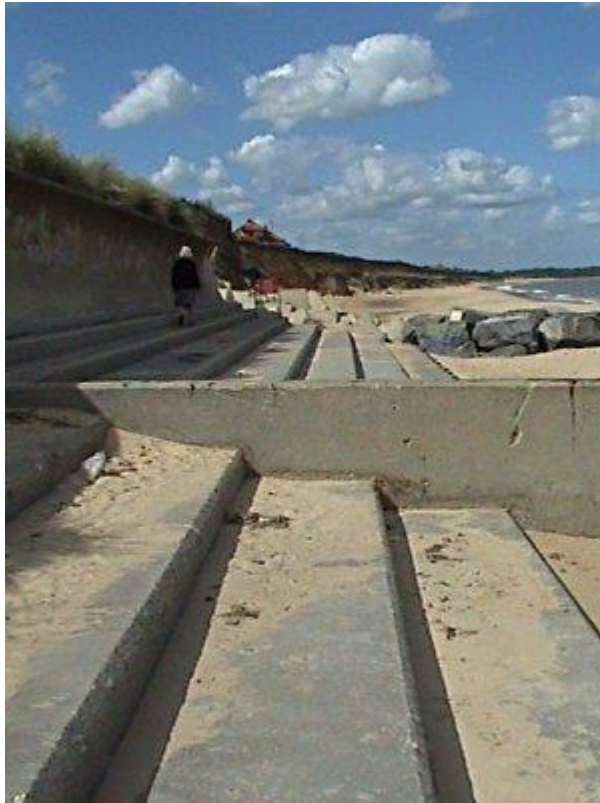
Northern end of sea defences at Easton Cliff; house on the cliff top is a few yards from the cliff edge
