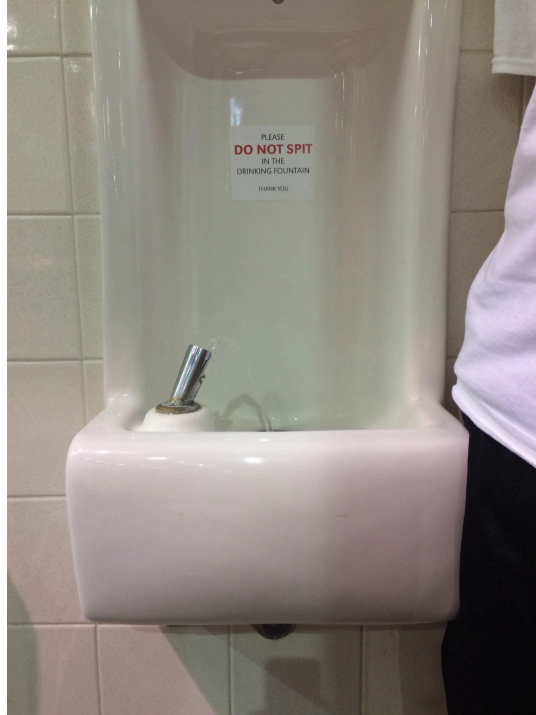
Rec - Room 153 Temp=21.5 C Stream=3 Height=2.5 Quality=2 Bottle Filling=2
