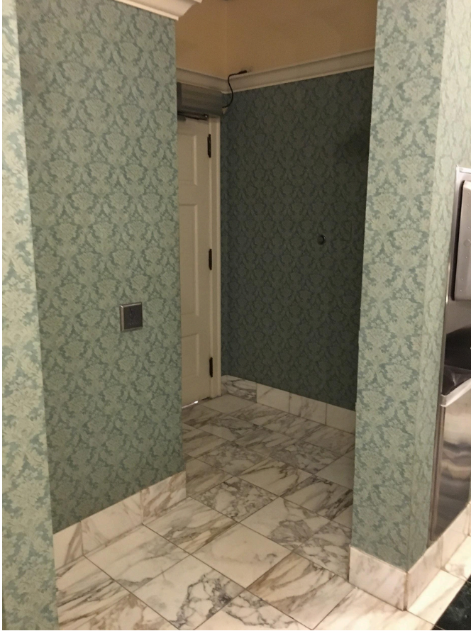
Image Description: Tight entryway to Hilton 4th floor restroom, requiring two 90 degree turns in a 30-inch pathway. The tile is white and gray marble, and the walls have a sage green brocade pattern.
