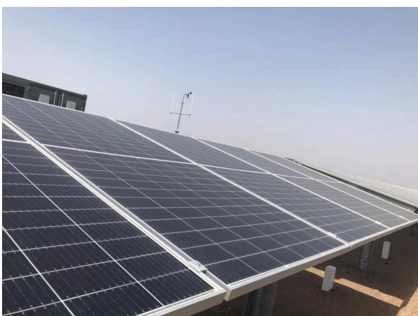
Figure 15: Solar panel array
