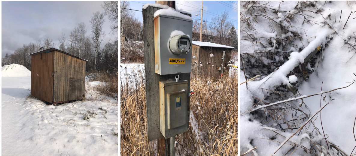
(Left to right) Chester Bowl pump house, power to pump house, and drain valves located near Kenwood Avenue, along service road.
