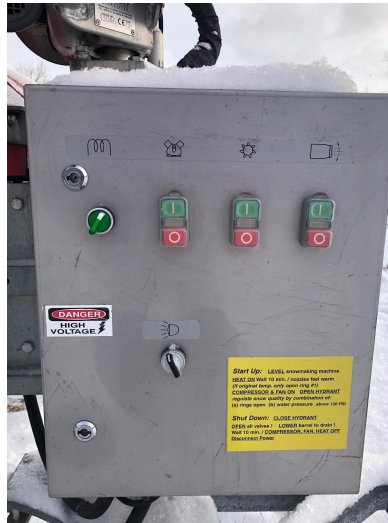
Control panel. Top row, left to right: heater (toggle switch), compressor, fan, oscillator. Bottom, search light (toggle switch)
