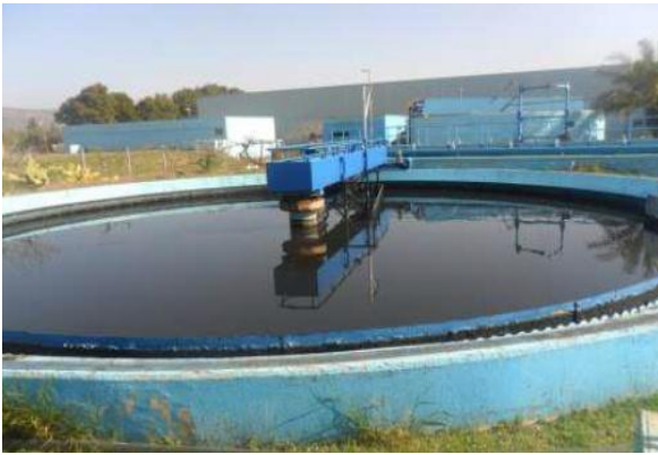
Figure 3a. Final clarification basin.
