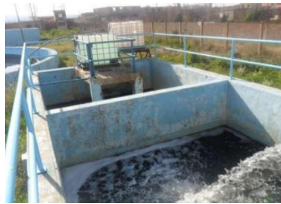
Figure 4b. Post chlorination basin.
