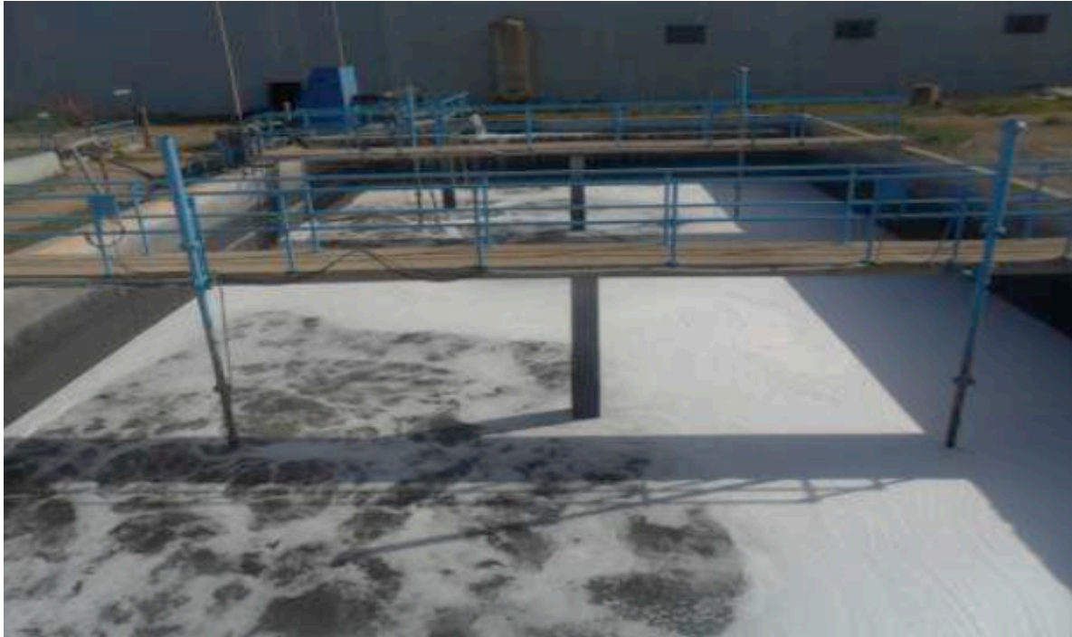
Figure 2. Photo of mixing and equalization basin N ° 1.
