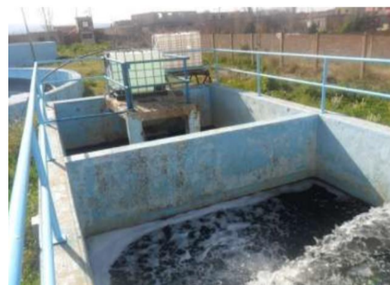
Figure 6b. Post chlorination basin.
