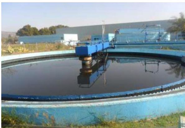
Figure 6a. Final clarification basin.
