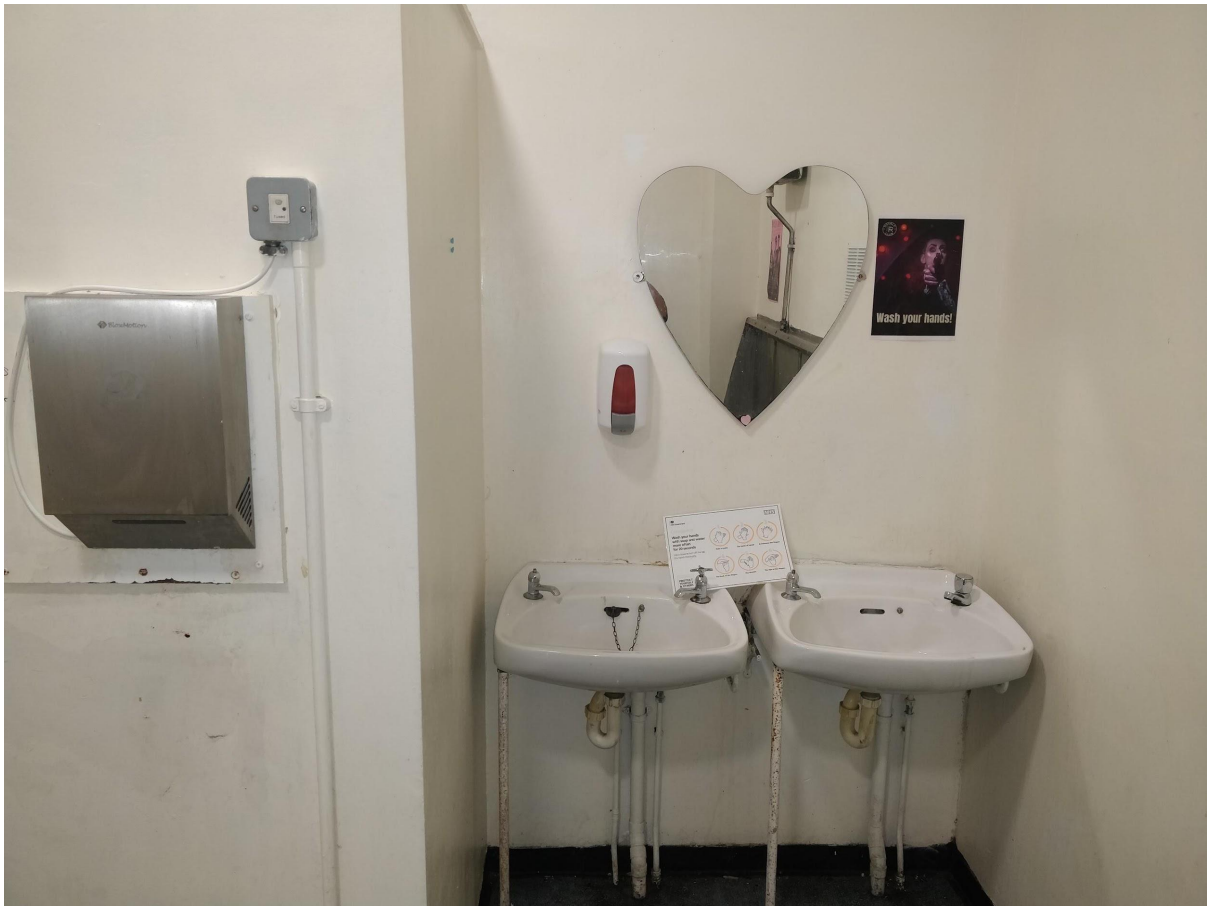
Image description: 2 sinks, with heart-shaped mirror and handsoap dispenser, all on wall with wall-mounted hand dryer on left of frame
