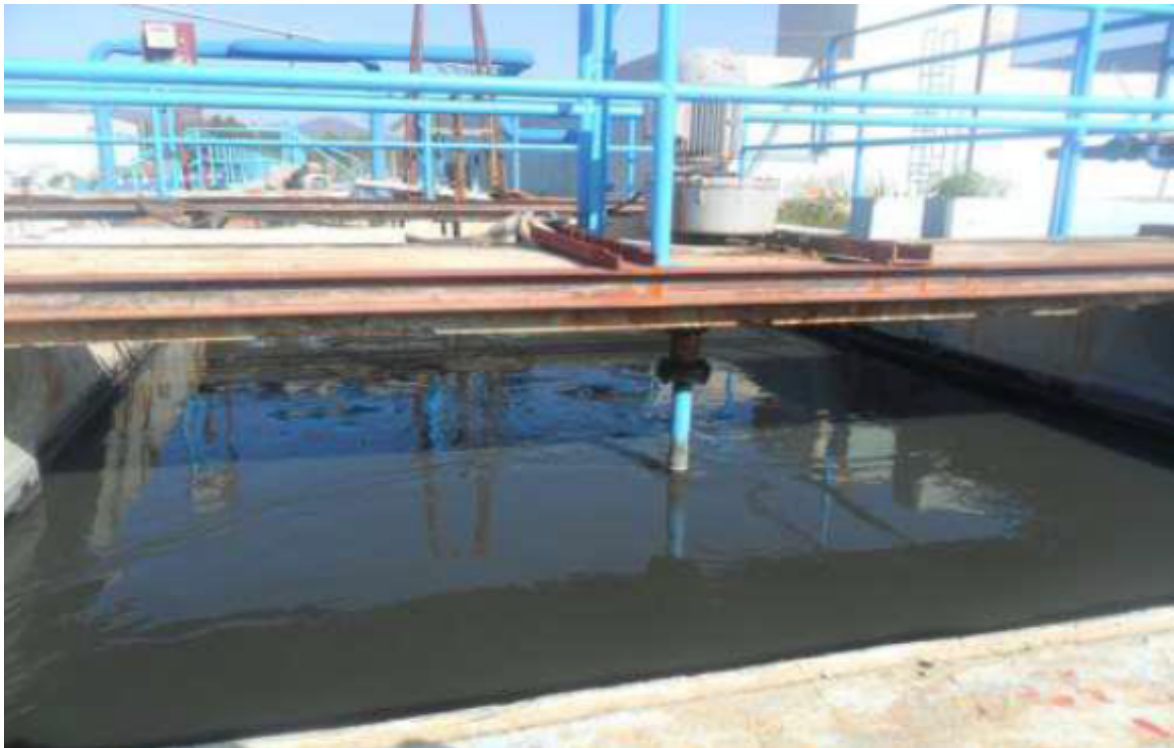
Figure 3. Mixing and neutralization basin N ° 2.
