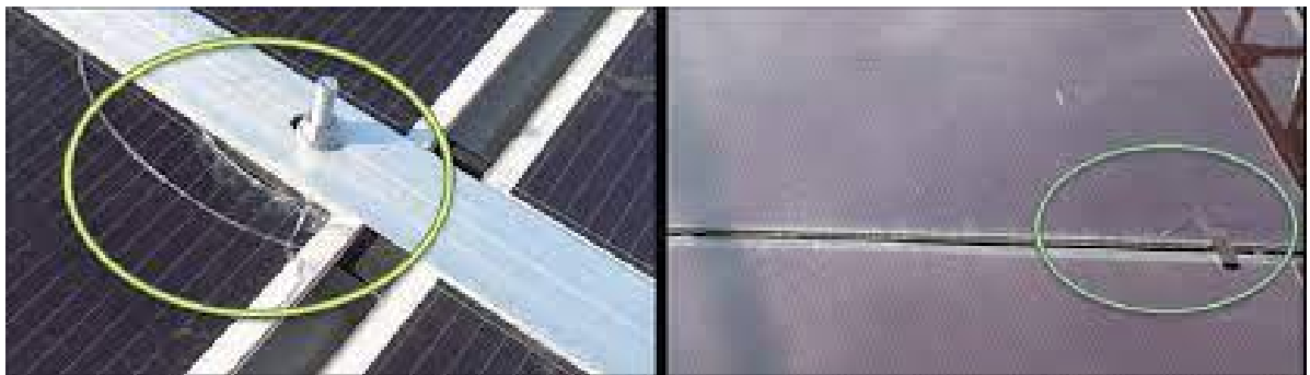
Figure 1-9: Left figure shows glass breakage caused by too tight screws and the right figure a PV module that broke due to poor clamp design [3]
