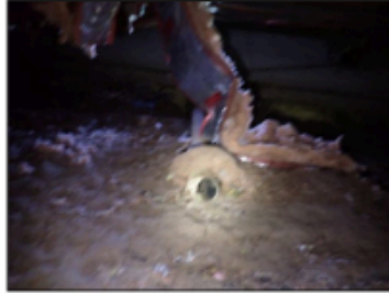
Makeshift drain noted.
