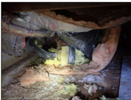
Damaged insulation noted.
