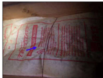
Insulation installed wrong side down
