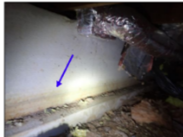
High water line noted.
