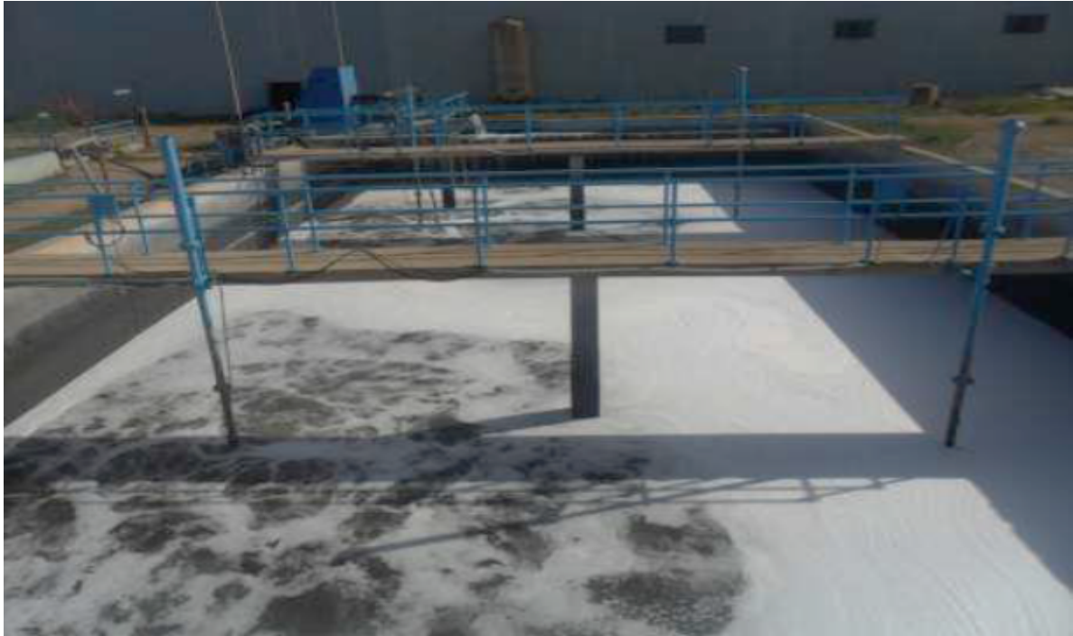
Figure 2. Photo of mixing and equalization basin N ° 1.
