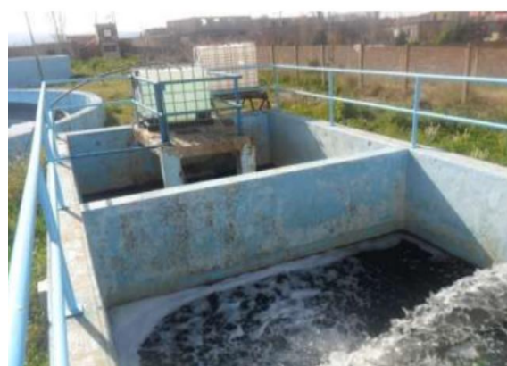
Figure 6b. Post chlorination basin.
