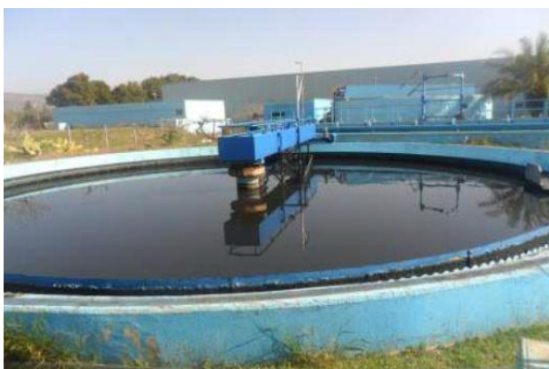
Figure 6a. Final clarification basin.
