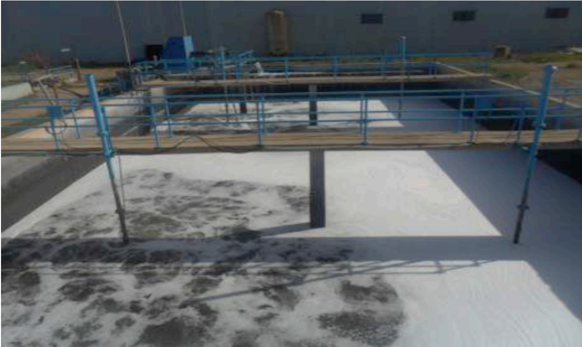
Figure 2. Photo of mixing and equalization basin N ° 1.
