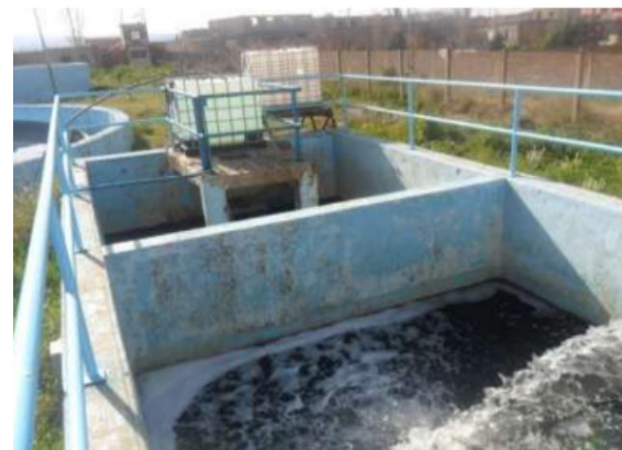
Figure 6b. Post chlorination basin.
