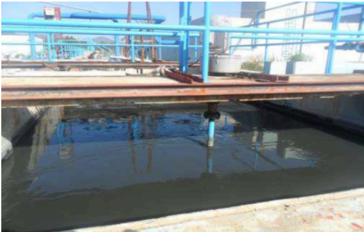
Figure 3. Mixing and neutralization basin N ° 2.
