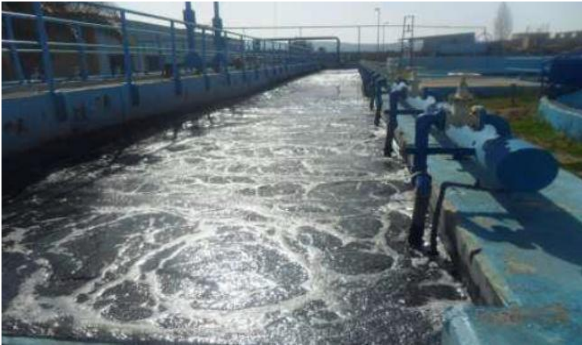
Figure 5. Biological basin (aeration basin).
