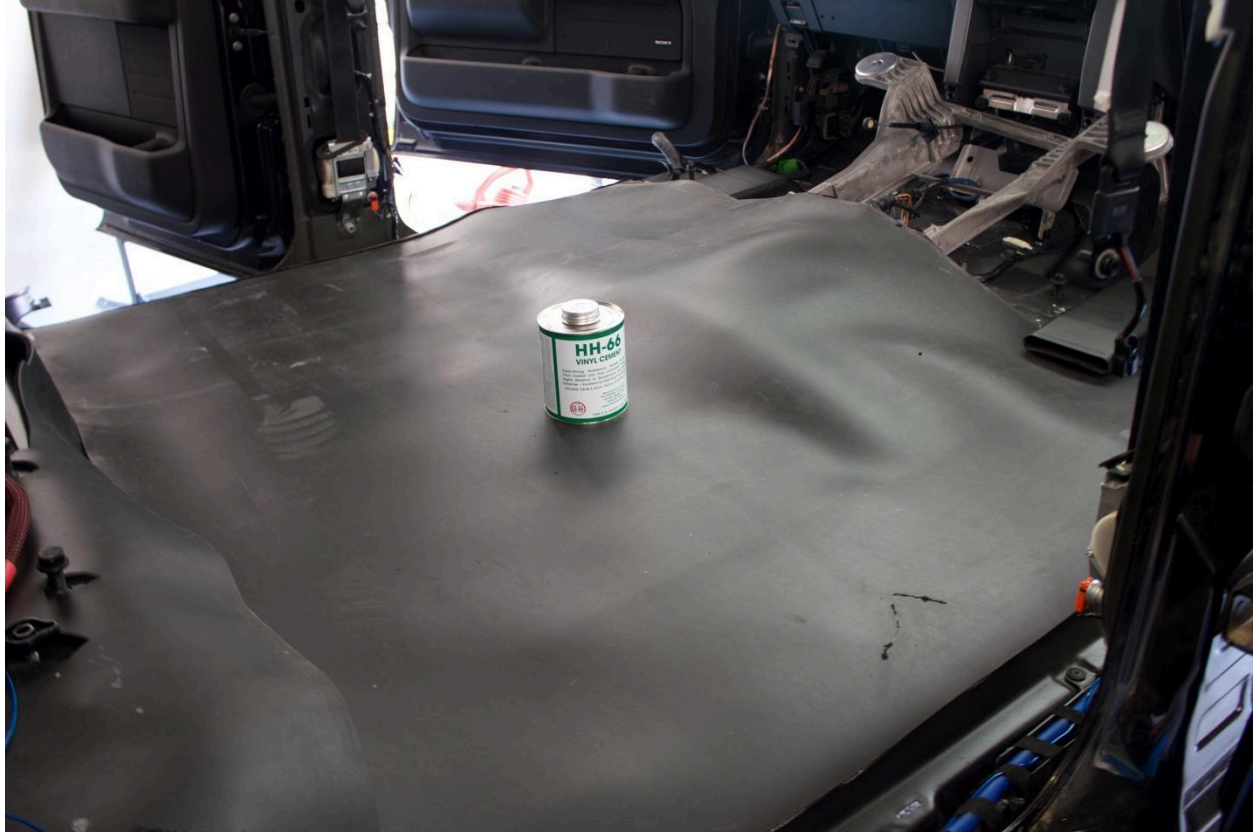
Place on the floor and seal to back seat platform piece using MLV and HH-66
