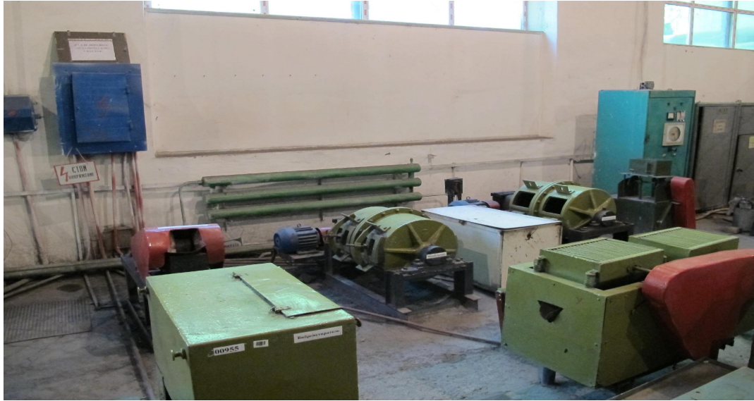
Section of crushing machines
