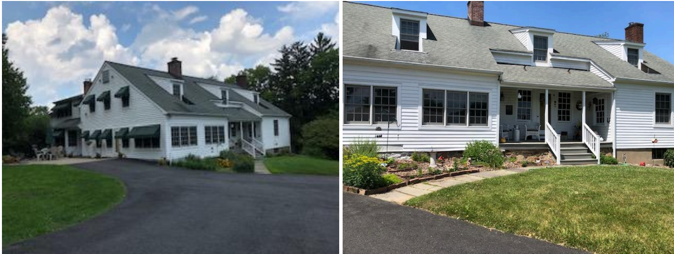
C. 1846 and later. 1 ½ story East Jersey Cottage. Built by Samuel Loree. House probably had a blacksmith shop on property. In the 1992 nomination cited as the “ Loree-Smith-King House. ” Fire damaged in the 1990s and rebuilt.
