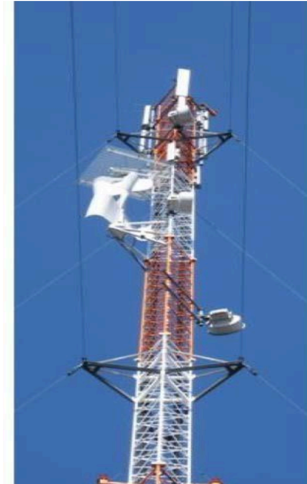
Figure 1-9: power cellular communication towers
