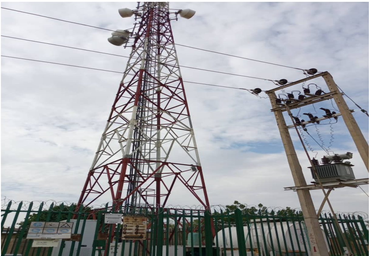
Cell tower in Madobi community (9mobile) with no guard at the time of visit – July 8, 2026 @ 4:35pm
