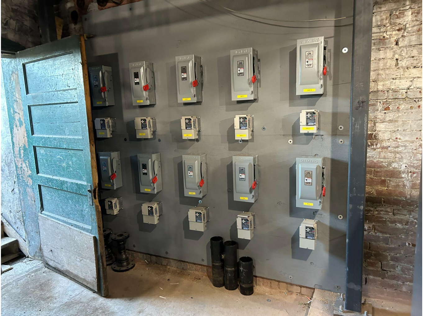
This picture is showing all of the disconnect switches and variable frequency drives (VFDs) that will control all of the pumps within the Boiler Room.
