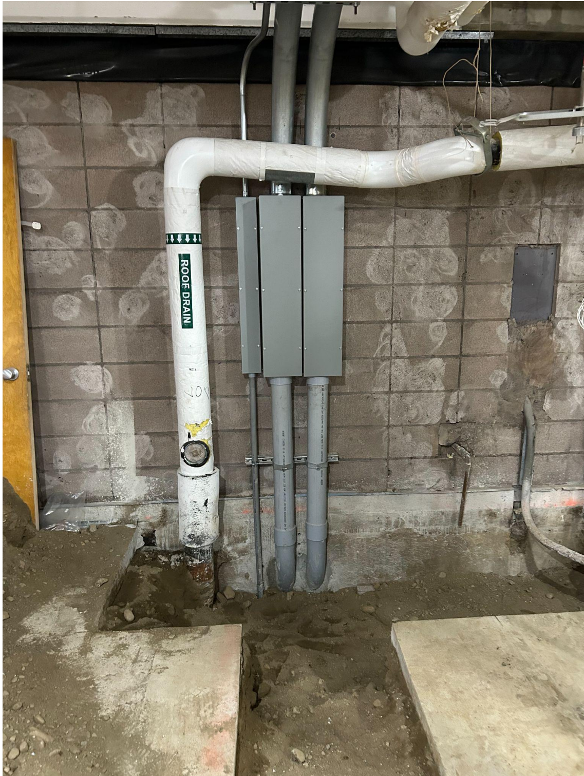
This picture is showing the electrical conduits that are coming from the new transformer that was installed last week. They come underground and this is how and where they transition from underground to then go overhead to the 1965 wing Electrical Room.
