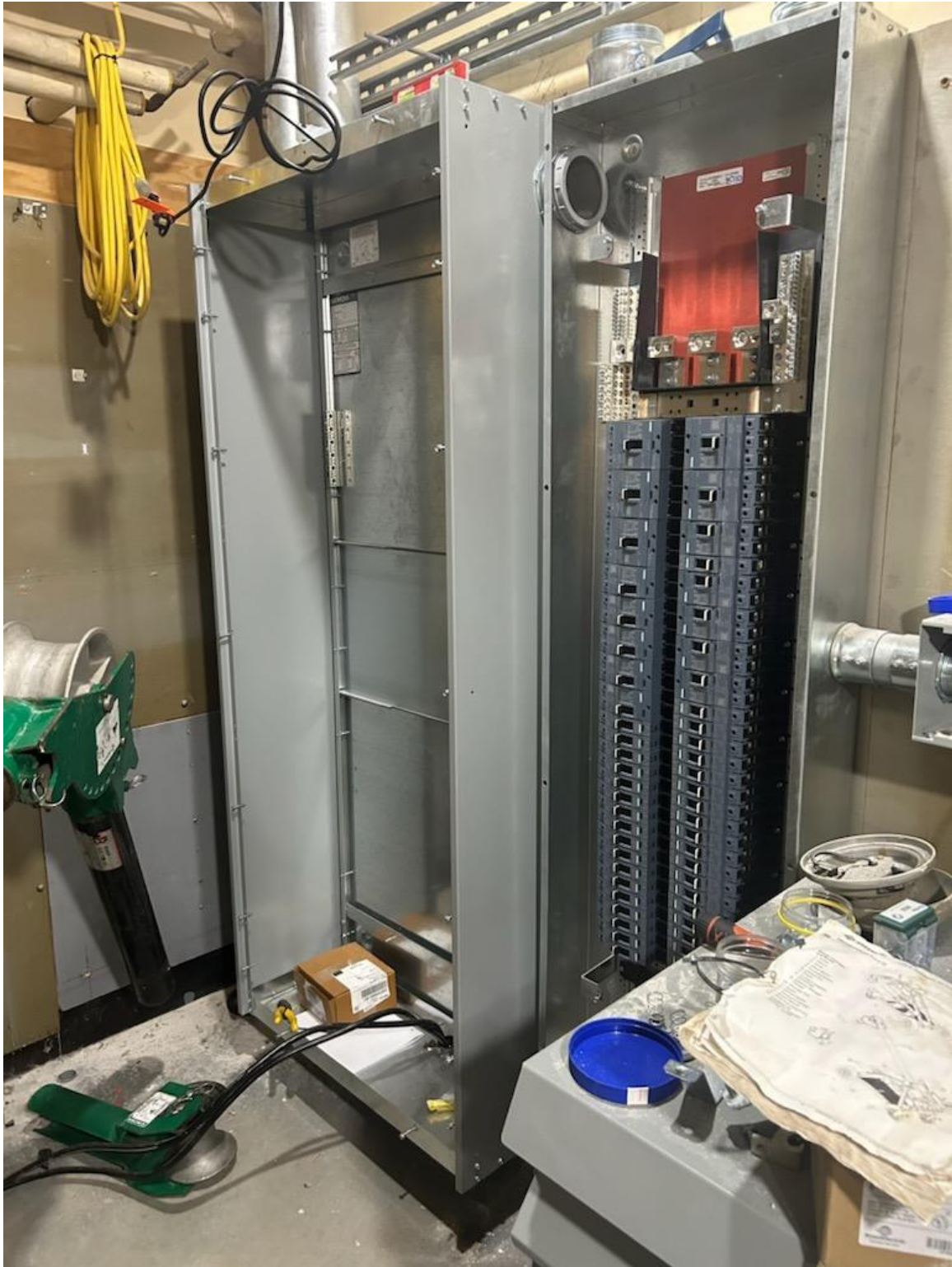
A picture showing where those main electrical conduits terminate. This is the new main electrical panel that is located in the Electrical Room within the 1965 wing of the building.
