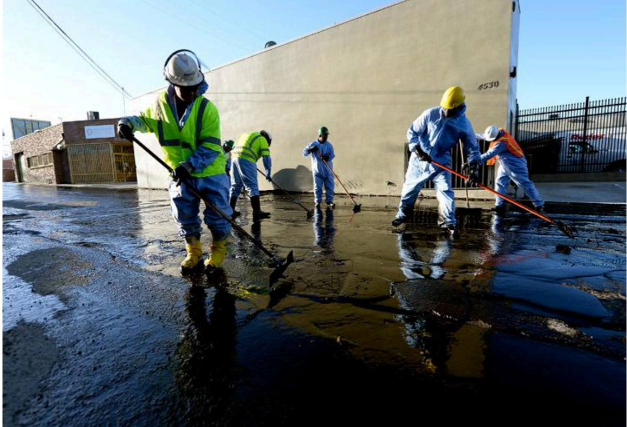
Figure 2: About 19,000 gallons of crude oil spilled into the street in eastern Los Angeles on May 15, 2014. It is believed to have been caused by valve failure, according to Plains All American Pipeline , who shut it off shortly after being contacted, but because the oil was under pressure, it continued to spill for 45 minutes.
