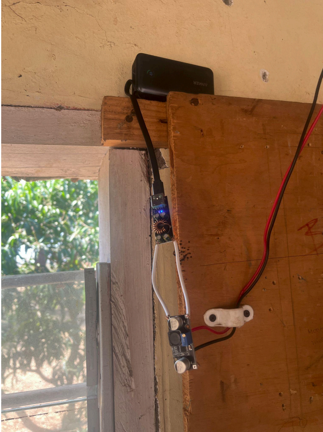
Simple Solar Charging
