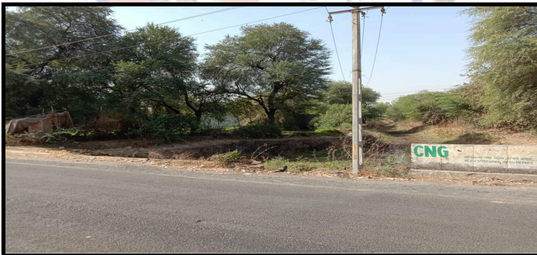
Figure 19 No fences are provided for safety against falling due to deep depression on the side of the road and center line is not provided
