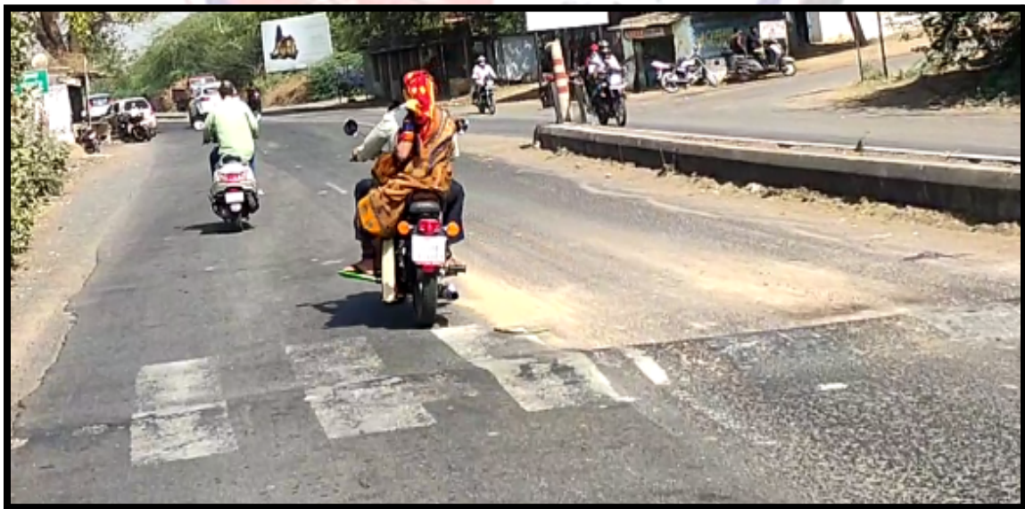
Figure 27 Bump width is less and not clearly visible, shoulder width not provided and polished aggregate
