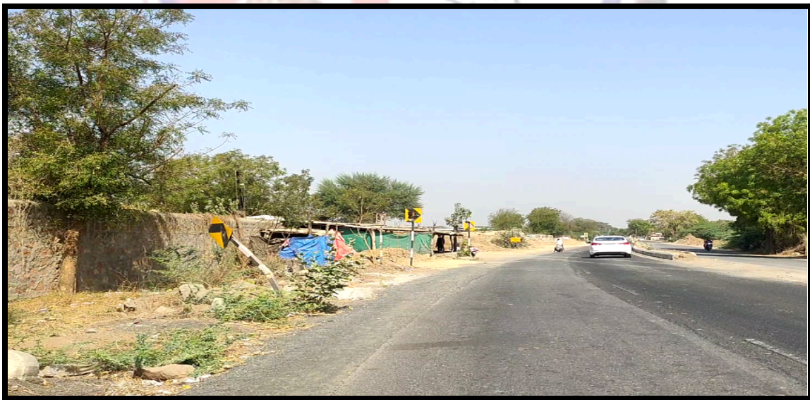
Figure 31 Signs are broken, center line is not clearly visible, shoulder width is not provided and road is poorly maintained as growing shrubs are reducing road width
