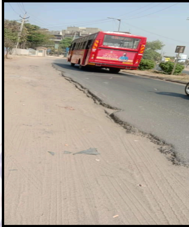
Figure 24 Shoulder width is not provided, reduced width for road due to side defects, edge cracking and no center line is provide
