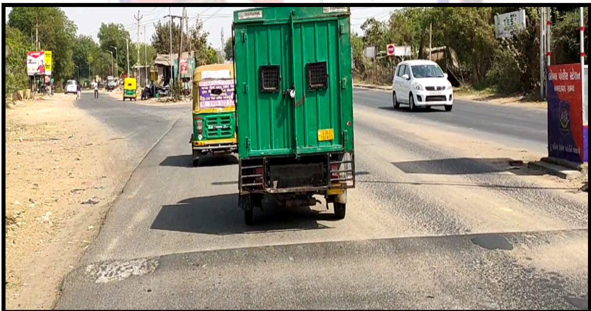
Figure 29 Bump marking is not provided, no intersection is provided at junction of road, no warning signals are provided
