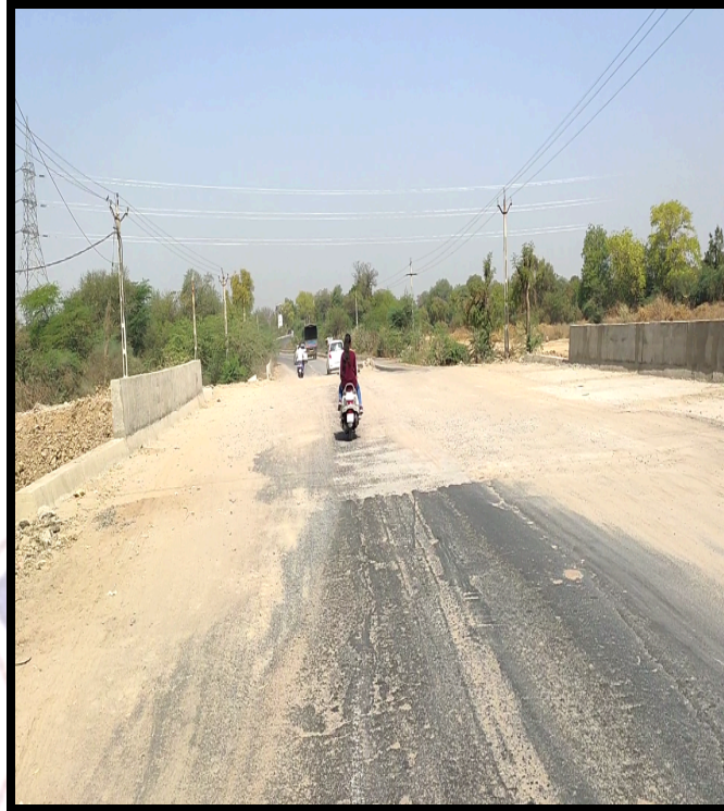
Figure 34 Poor road condition with depression and loose sand on the road which reduces skid resistance
