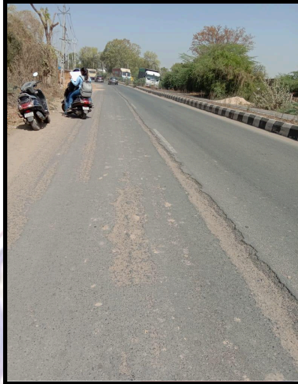
Figure 20 Longitudinal cracking and uneven alignment of road
