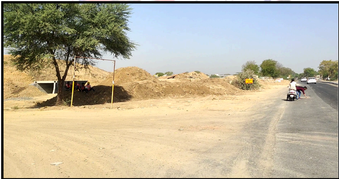
Figure 35 No protection of steel sheets provided on the road side construction site, no cautionary signs are provided and center line and shoulder width are absent
