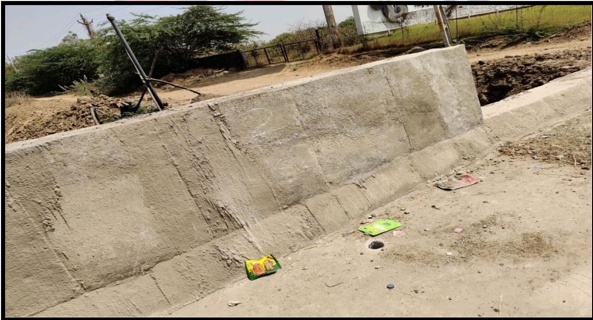
Figure 33 Fences are not provided for the full length of the depression due to which part of deep depression is open which can be prone to falling of the vehicle
