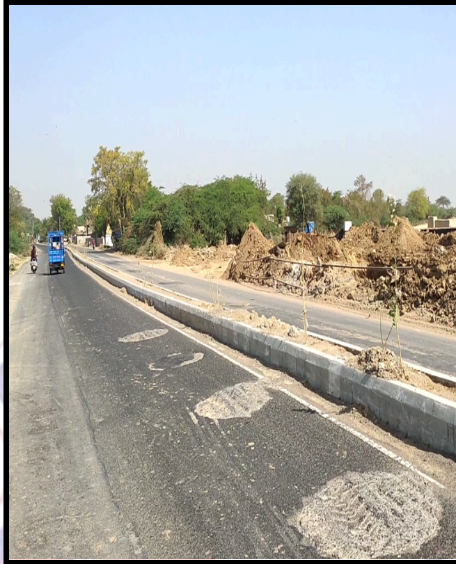
Figure 26 Defective pavement, no center line and shoulder width is provided
