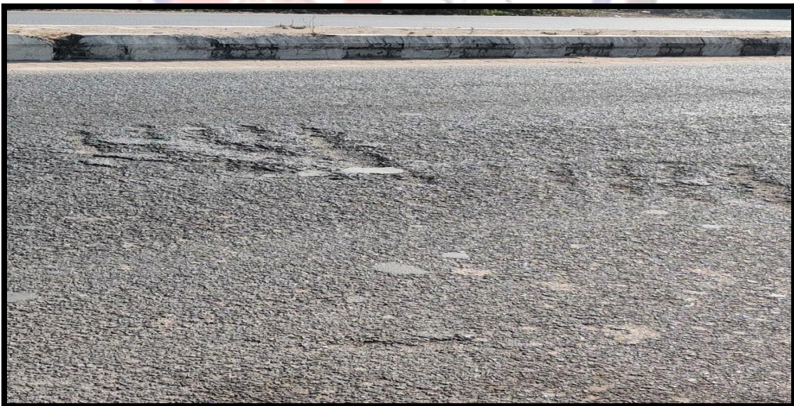
Figure 25 Raveling of pavement, center line is not clearly visible
