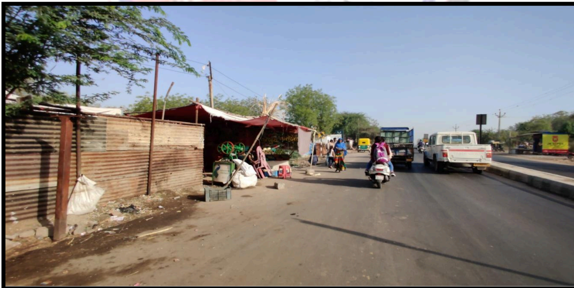
Figure 37 Shoulder width and center line are not provided and illegal shops on road sides reduces road width
