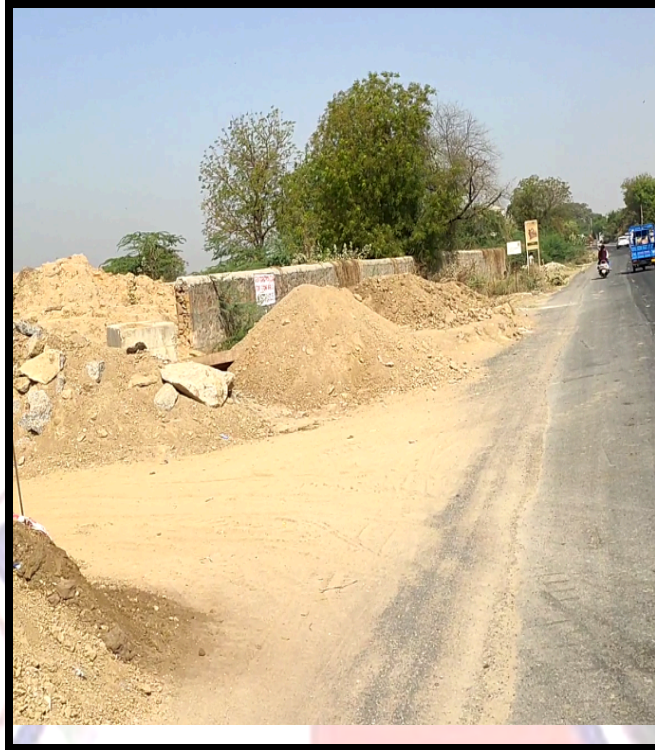
Figure 28 Loose construction materials of the site are stacked on the road without protection and shoulder width is not provided
