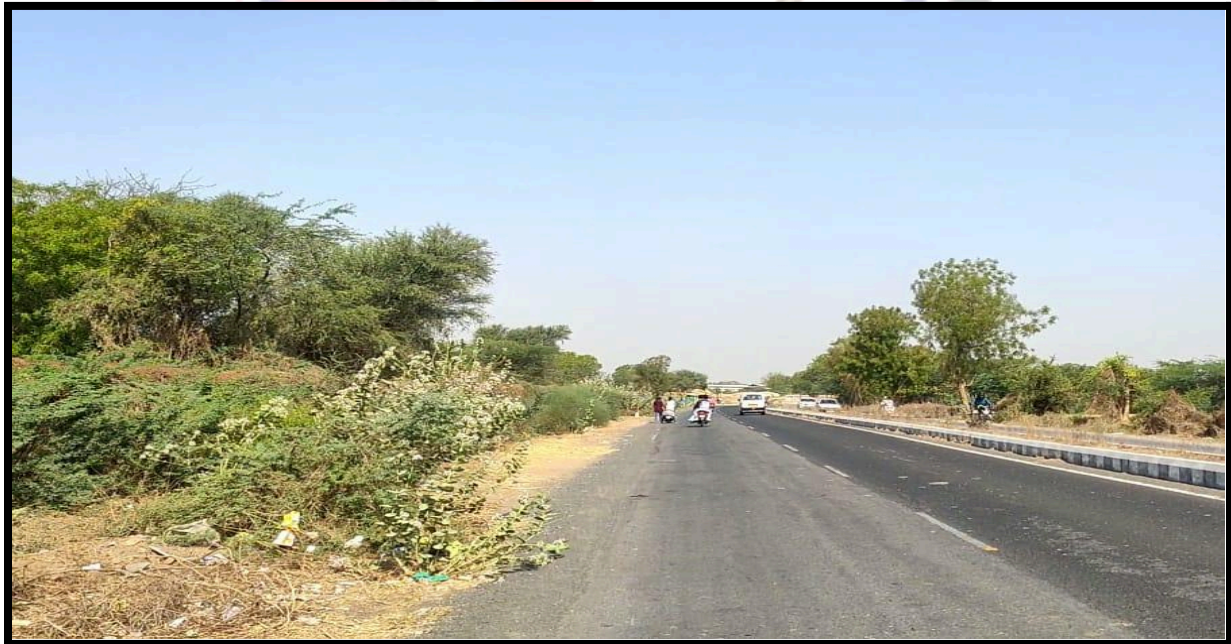
Figure 39 Guard rails for safety against trees is not provided, Shoulder width is not provided, uneven road surface, Center line width is improper
