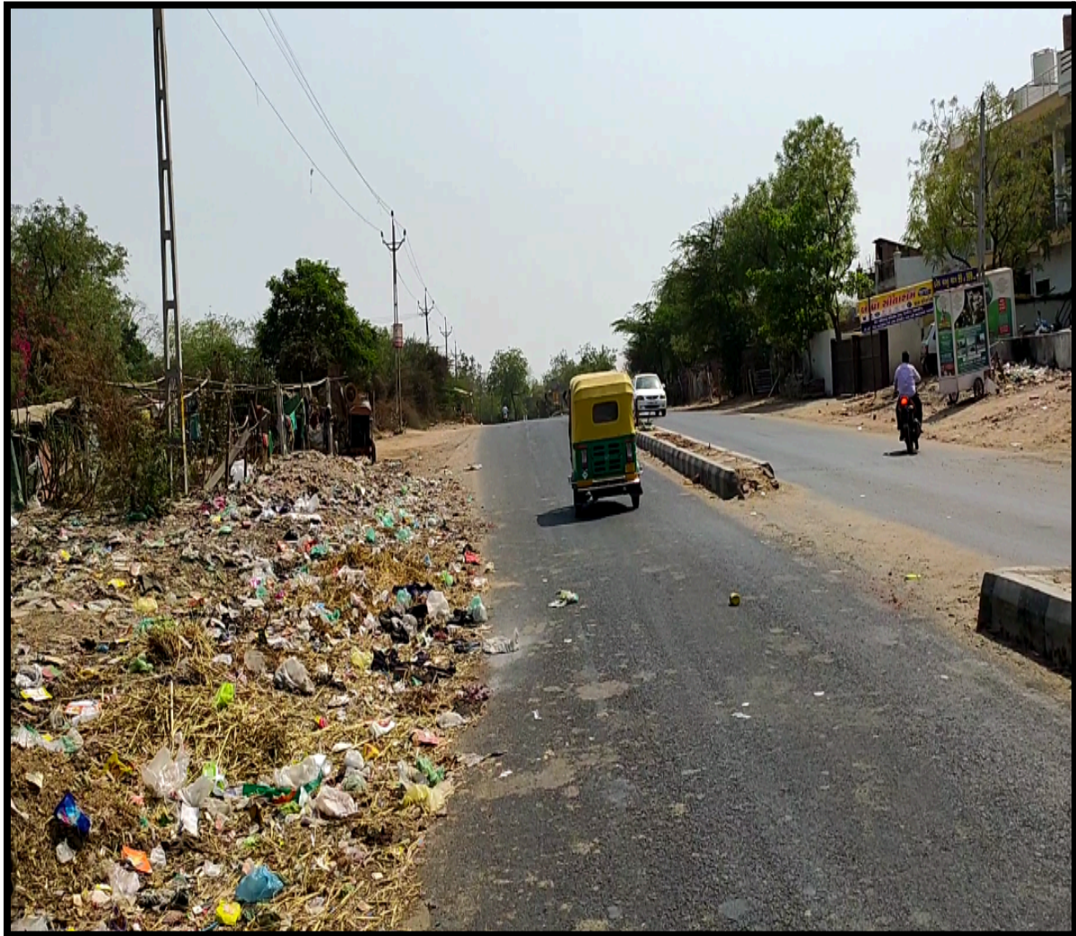
Figure 17 Garbage accumulation on side of the reduces width of the road and due to it shoulder width is not visible, center is not provided and damaged median
