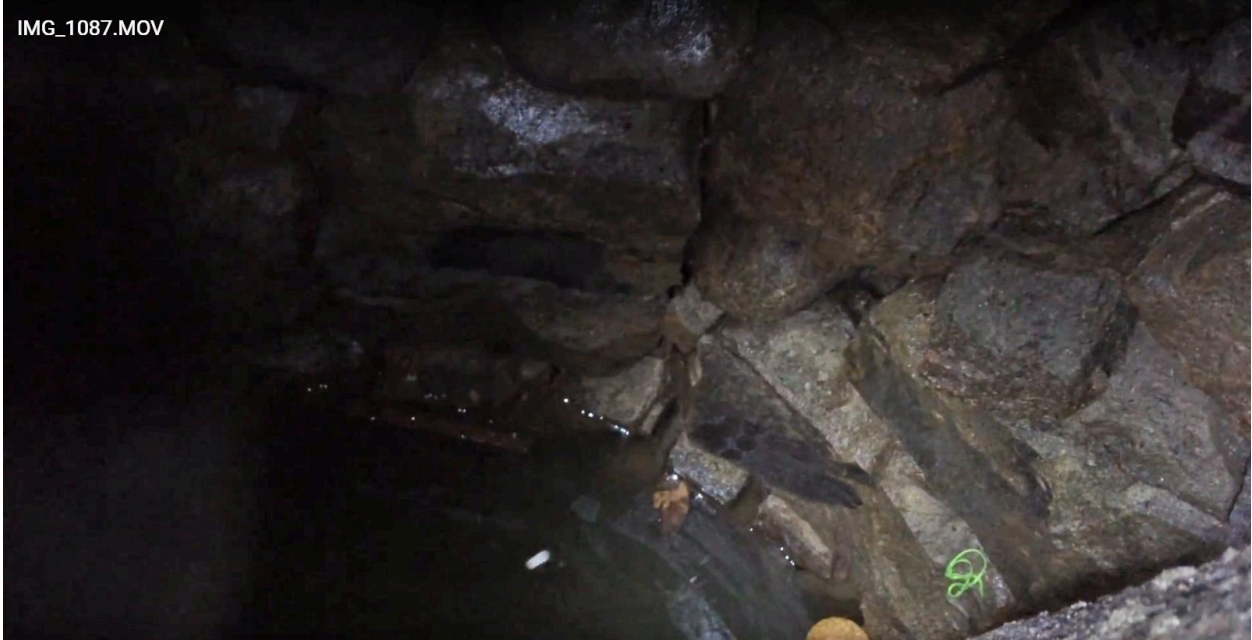
Figure 31- View near bottom of well showing water pooling at the bottom. Green string fell in from recent landscape work, as did the fall leaves (Photo taken in October). Pipe is visible in extreme lower right of image. View is approximately 3 feet wide.
