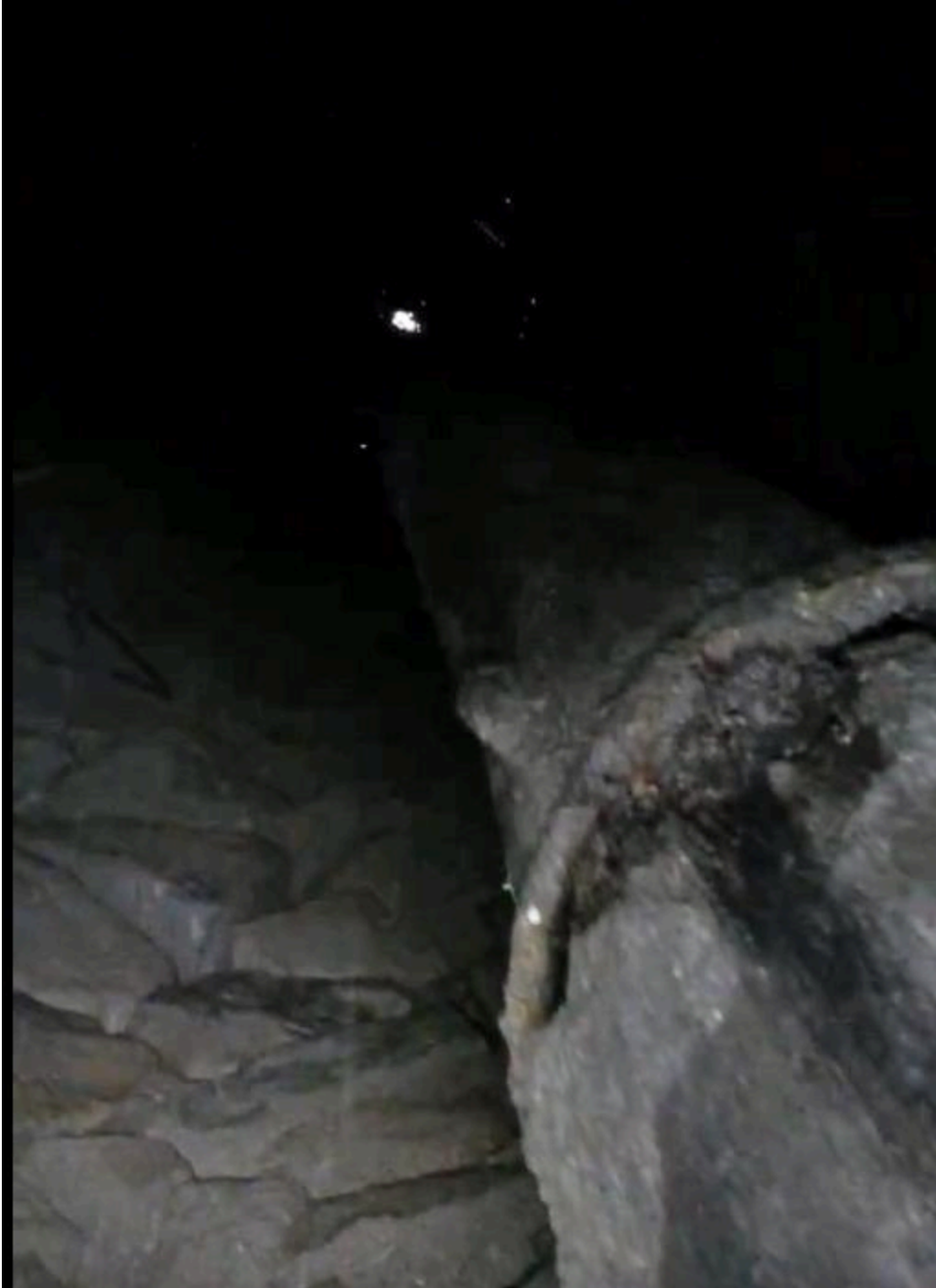
Figure 35- Banded coupling between the lower and upper pipe segment. Pipe is approximately 10 inches wide. View facing downward.
