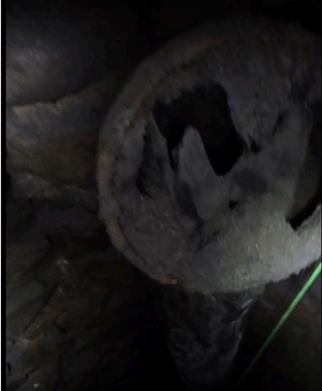
Figure 34- Detailed view jagged upper/top end of pipe segment with iron band remaining, but hanging off of the broken element. Green string from landscapers. Pipe is approximately 10 inches wide. View facing approximately horizontal in well.
