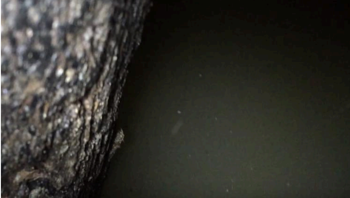
Figure 32- Video still of the water at the bottom of the well showing its lack of transparency. Pipe to the left.
