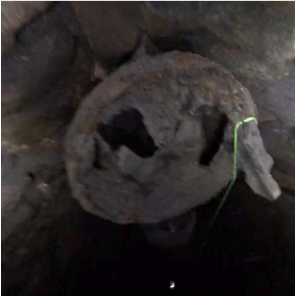
Figure 33- Full view of upper coupling. View facing slightly downward in well. Pipe is approximately 10 inches wide.
