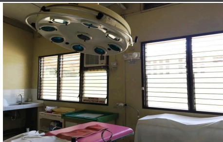
Delivery room light
