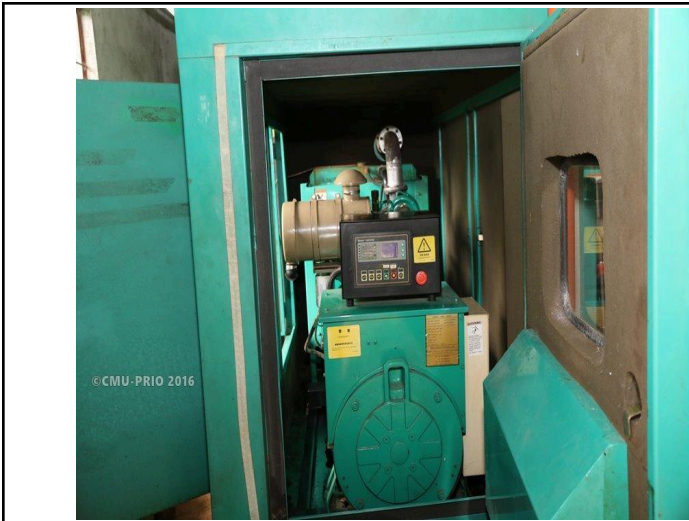
Standby Generator Set
