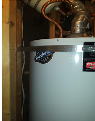
Image showing: water heater secured to the beams.
