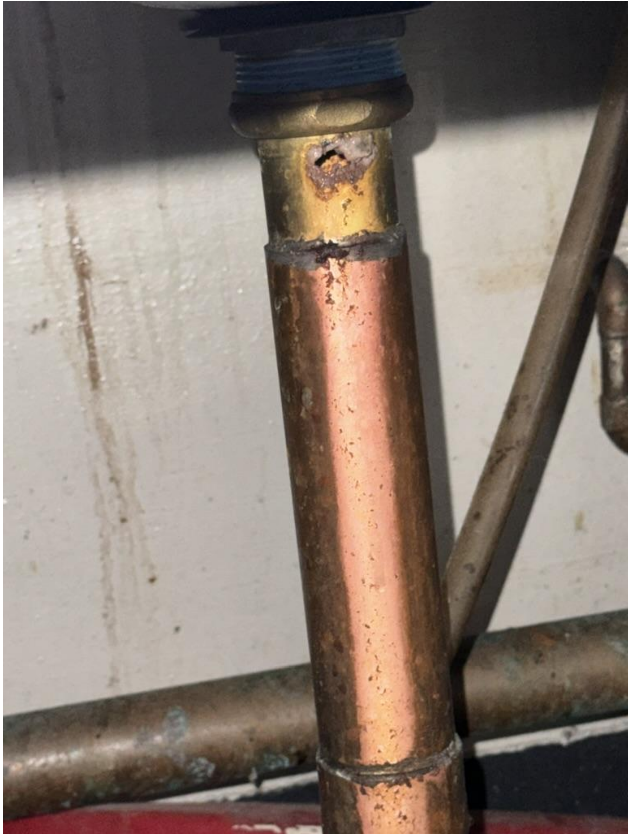
Pipe in Question
