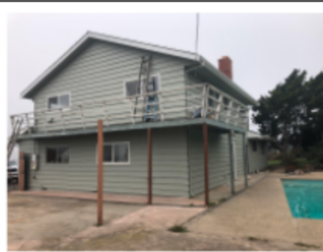
Home with the defective deck during preparation for sale in September 2020.
