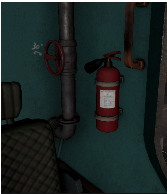
Valve and Extinguisher
