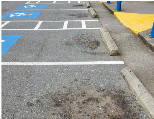
Photo 2: Stained parking spaces
